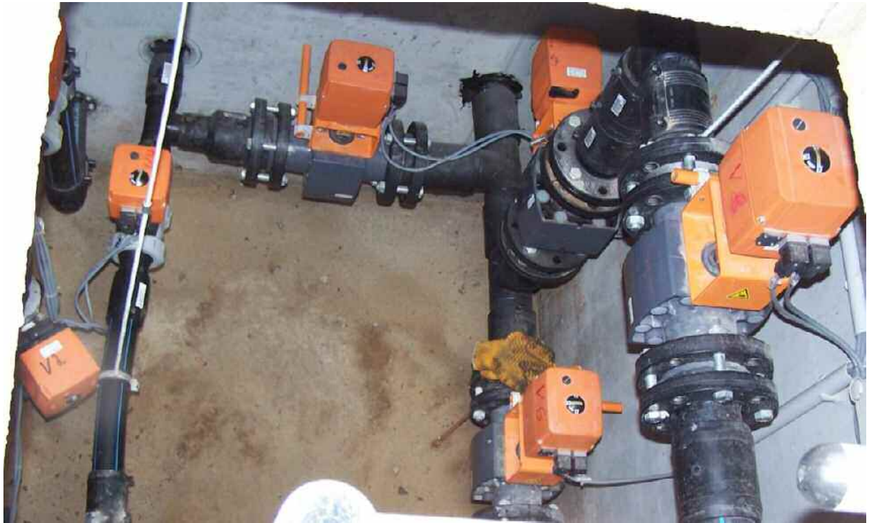
Figure 2 An additional fitting shaft ensures the redundancy of the plant components for watering
